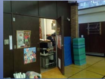
SCHOFIELD: Gym Closet Office Ventilation
